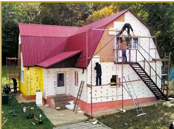
Before snow fell, believers from Europe helped apply insulation to the Rehabilitation Center near Ternopil. Now the building is snug and more energy efficient.
